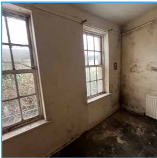
Examples damp plasterwork prior to commencement of the works
