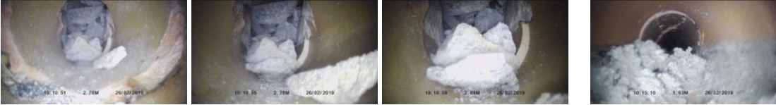
Debris, appears to have been blocked off
