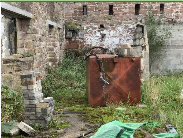
P3: Inside the derelict barn
