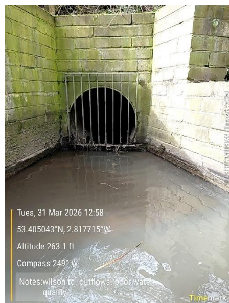
Photo 11: Outflow, poor water quality (SJ 45734 90114)
