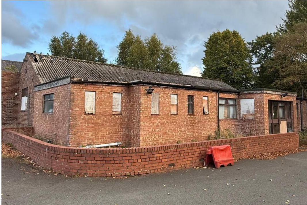
3. Major gaps in corrugated roofing sheets
