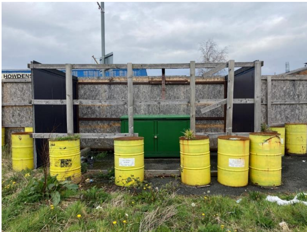
PLATE 4 ELECTRICITY BOX IN NORTH WEST CORNER OF SITE
