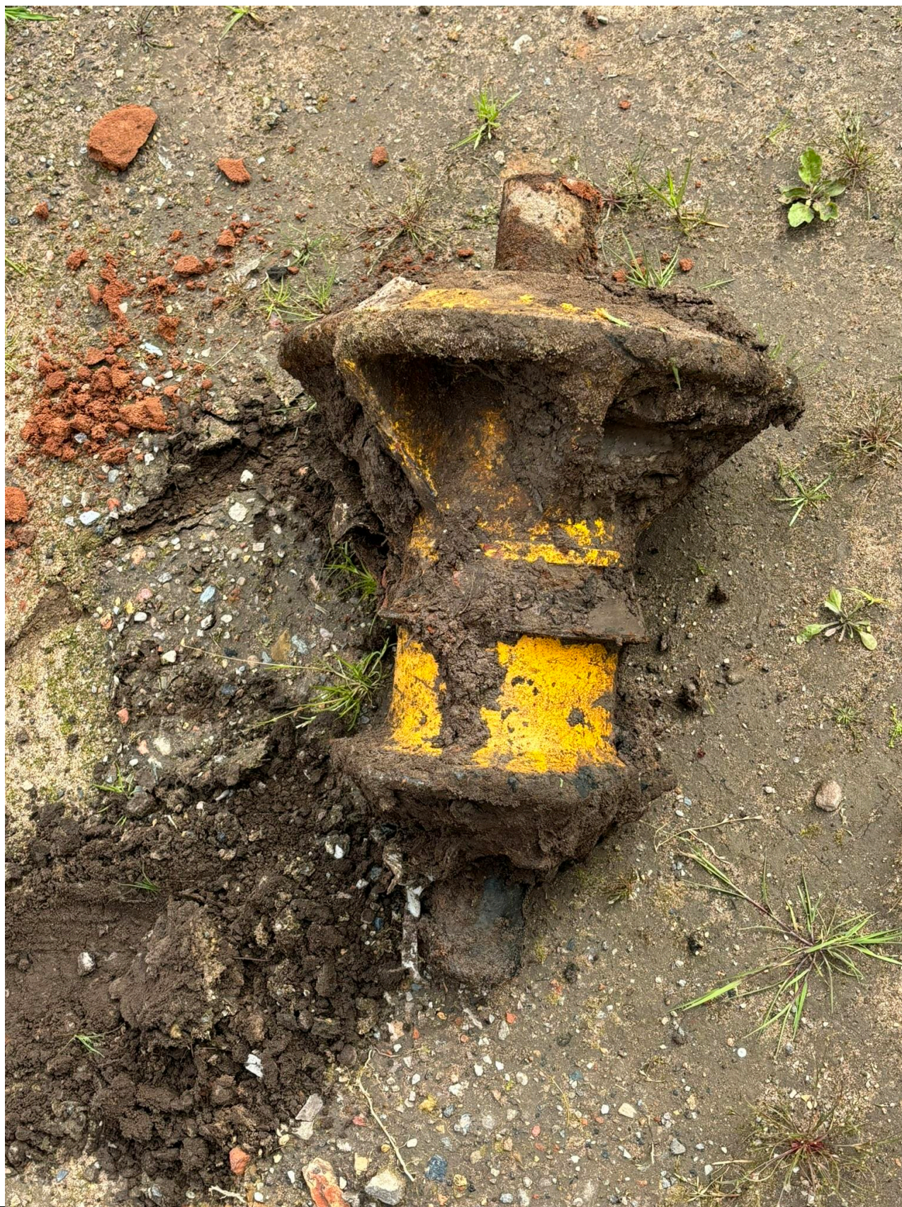
Plate 13: TP12 obstruction found during the excavation
