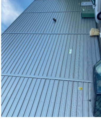
Existing Ventilation Louvre
