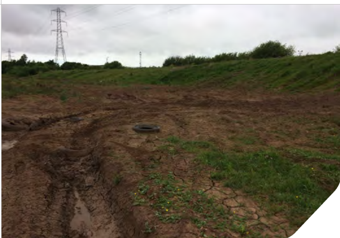
Photo 03: Showing rutting near site entrance and earth bund along northern boundary
