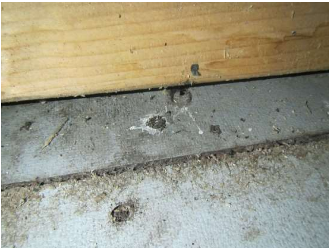
Photograph 12 – Bird droppings found within Building 1.
