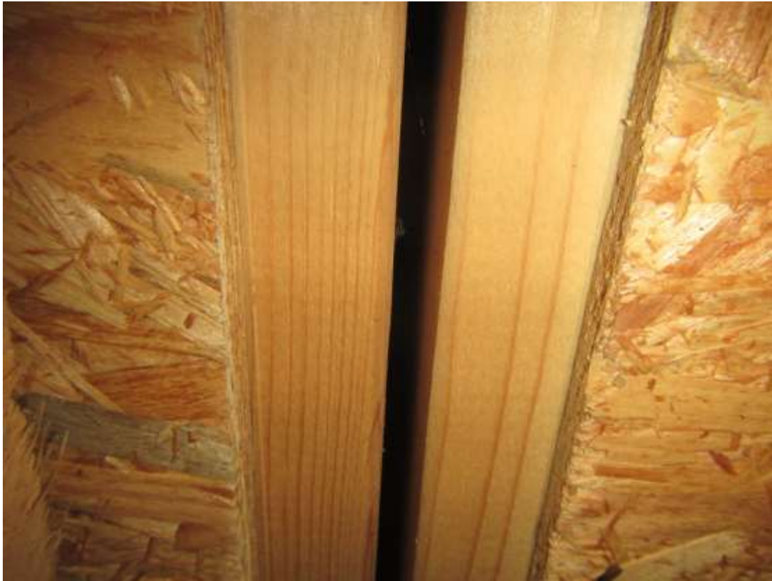
Photograph 11 – Superficial cavities in between the woodwork in Building 1.
