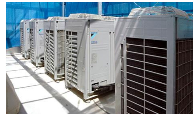
Figure 10: ASHP external unit
