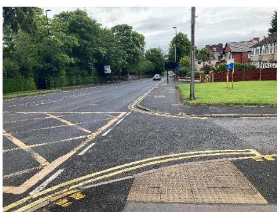
Photograph 5: Tactile Paving and footway conditions at the site frontage viewing eastbound along Huyton Lane
