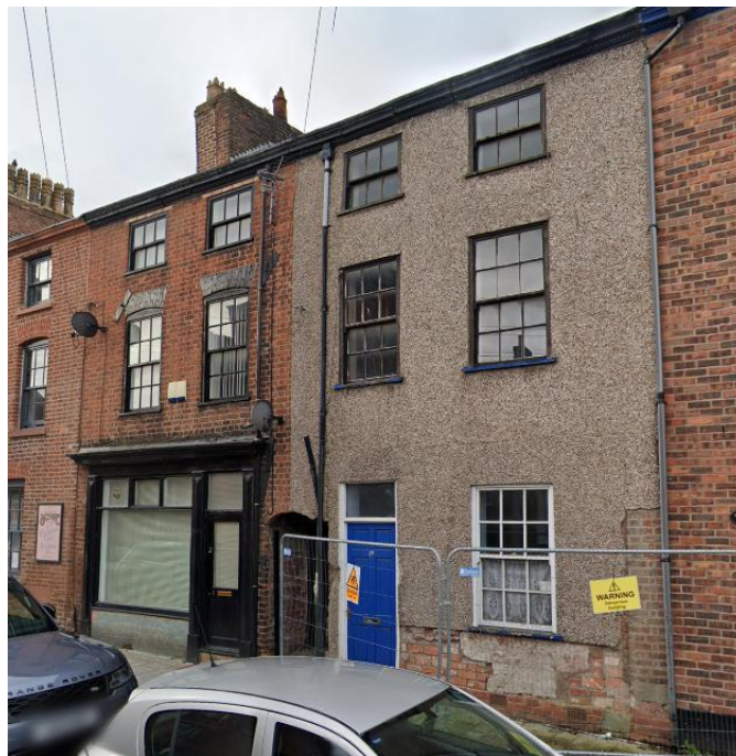
17 Atherton Street (Black shop Frontage) and 19 Atherton Street (Blue door, damaged frontage, surrounded by safety fencing)
