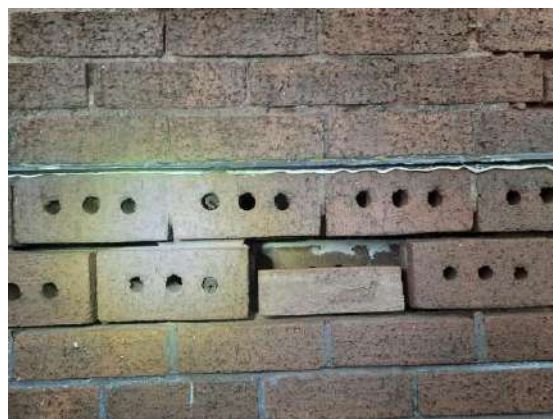
Plate 4.9: Gaps in Brickwork on South-west Side of Rooftop Brick Structure.
