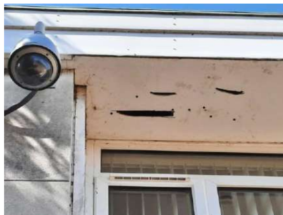
Plate 4.7: Damaged Soffit Boarding on Southern Elevation of Section 1 of Building B4.
