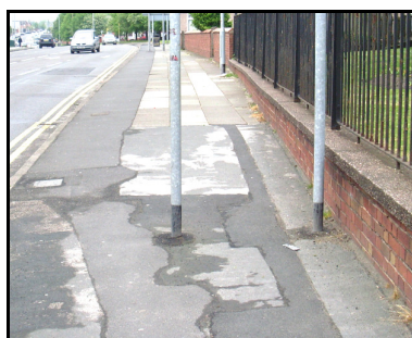
Photograph 1: Condition of footway
