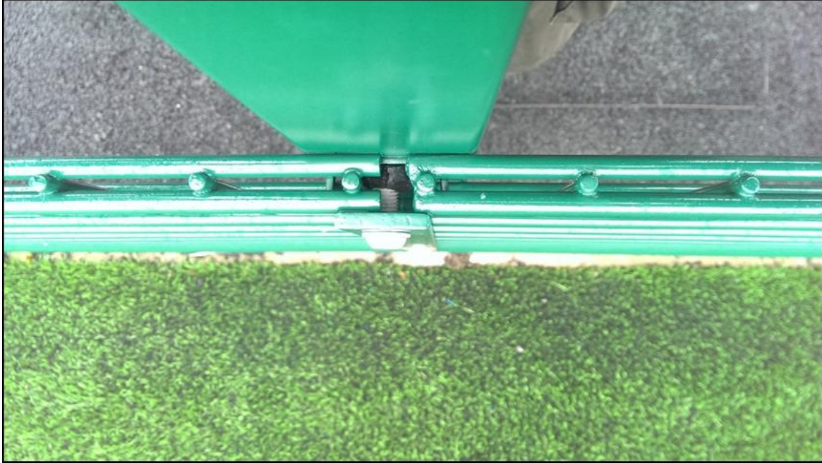
Figure 11: Image showing neoprene isolators
