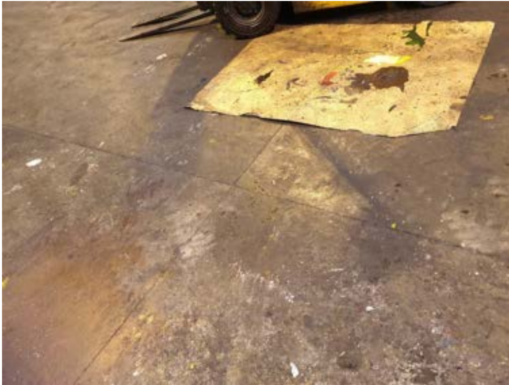
Photo 15: Floor of middle building showing spillages and floor joints.
