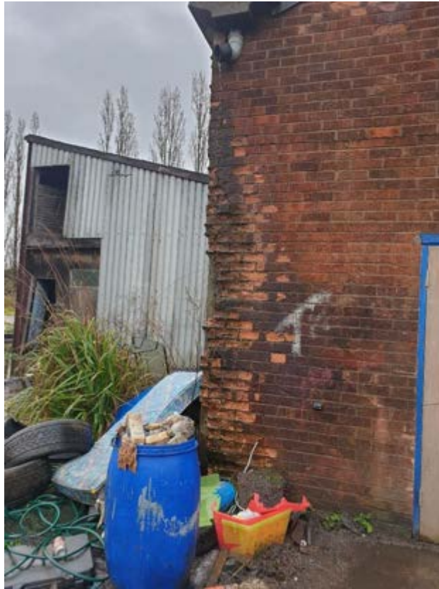
Photo 3: View of lean-to adjoining large building (looking NE), showing poor condition of brickwork.
