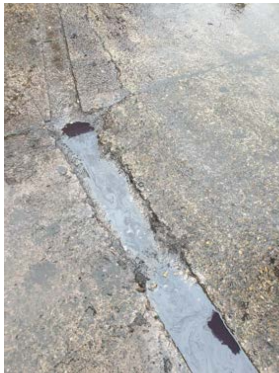
Photo 50: View of ink within surface water on site, approximate location is outside the most southern large building.
