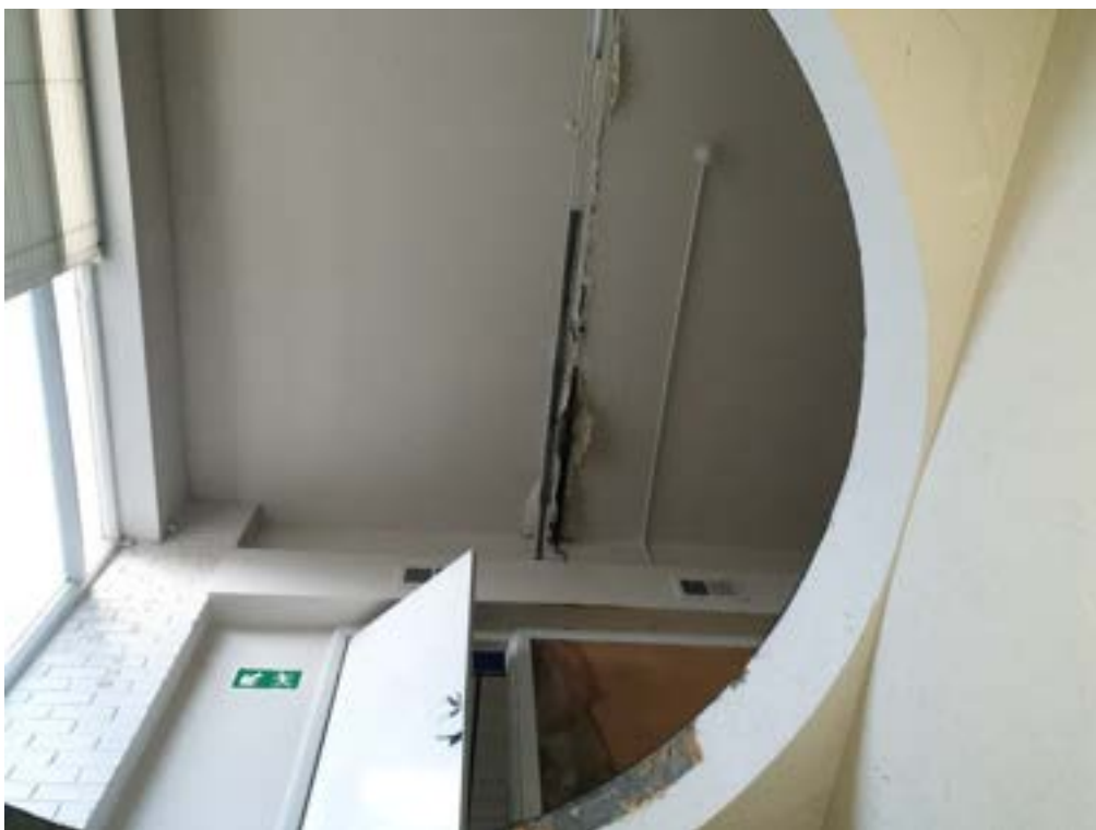
Photo 18: View of damaged roof in the west area of the most southerly building.
