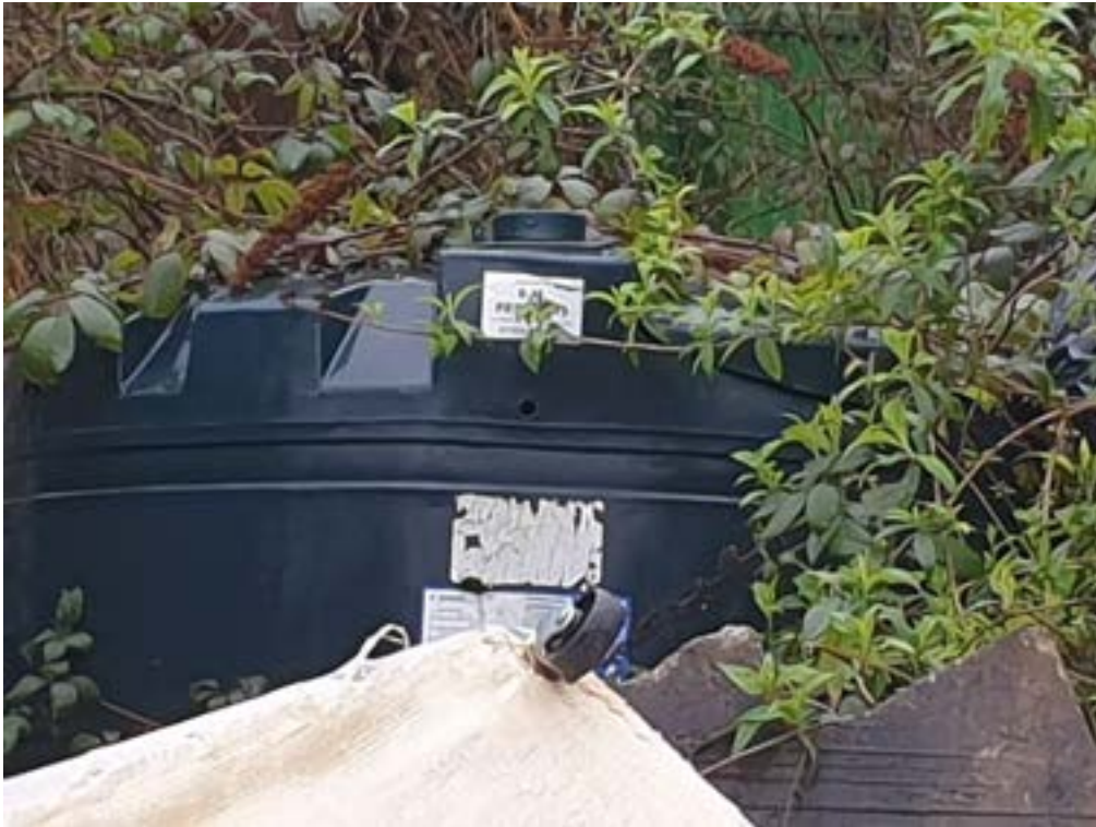
Photo 37: Close-up view of fuel tank located in NW of site.
