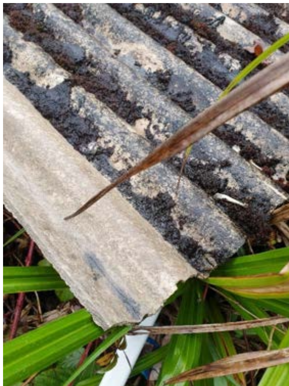
Photo 36: Close-up view of asbestos sheet found in NW of site.
