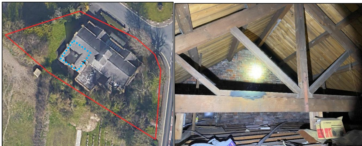
Figure 4.2 – Location of loft space (left) and character of the loft space (right)
