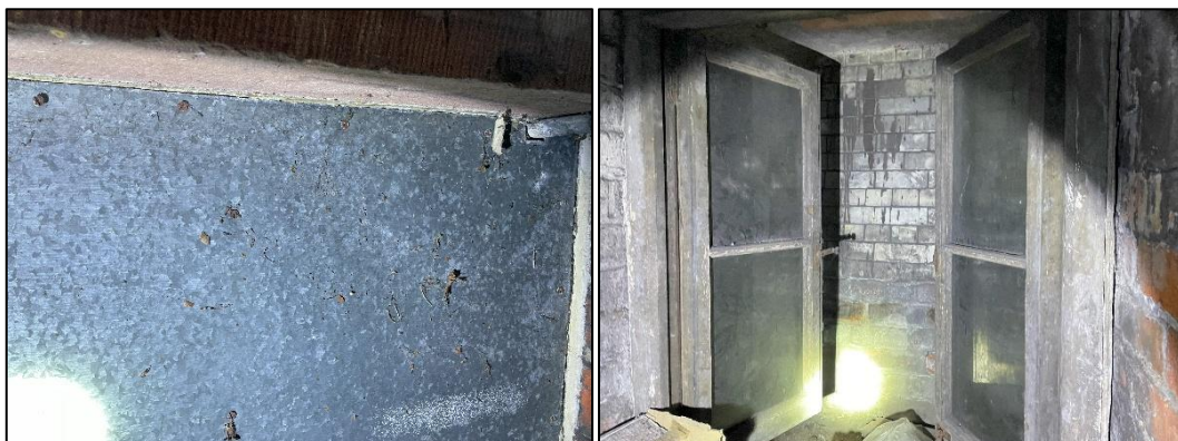
Figure 4.5 – Steel sheeting over cellar window (left) and second window leading nowhere (right)
