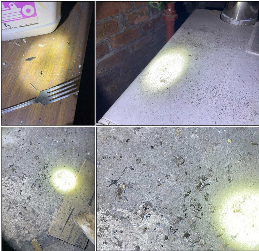
Figure 4.6 – Bat dropping attributable to pipistrelle bat (top left), dropping residue on white goods (top right), mixed droppings on floor (bottom left) and zoomed image showing mix of pipistrelle and brown long-eared droppings, displaying crumbly and/or mouldy state (bottom right)
