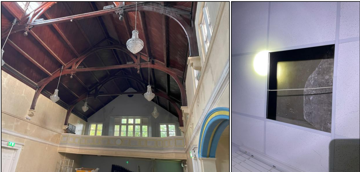
Figure 4.1 – Character of the hall with vaulted ceiling (left) and flat roofed extension with false ceiling (right)
