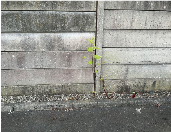
Plate 9.7: Small Number of Japanese Knotweed Plants Along South-east Boundary of Ambulance Station.
