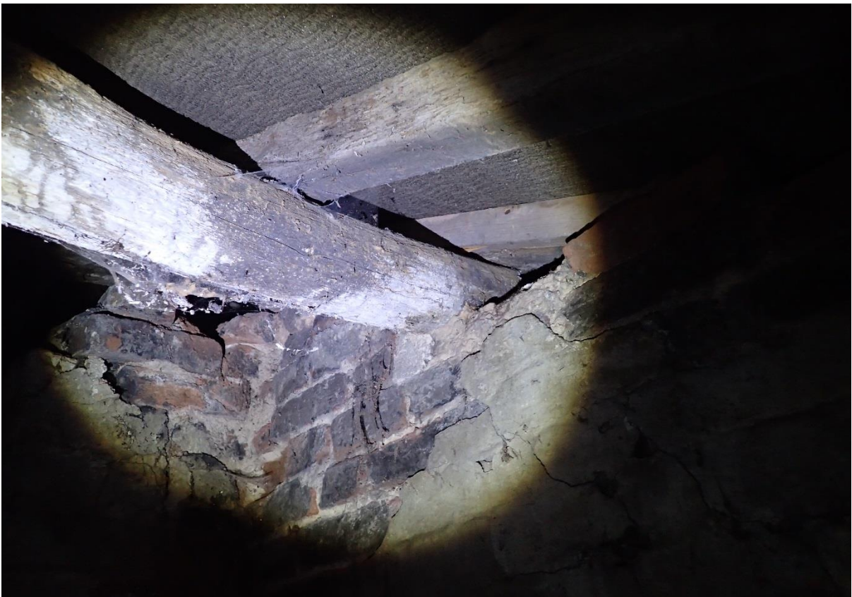
Photograph No. 4 – Close up of purlin with evidence of woodworm and beetle attack.
