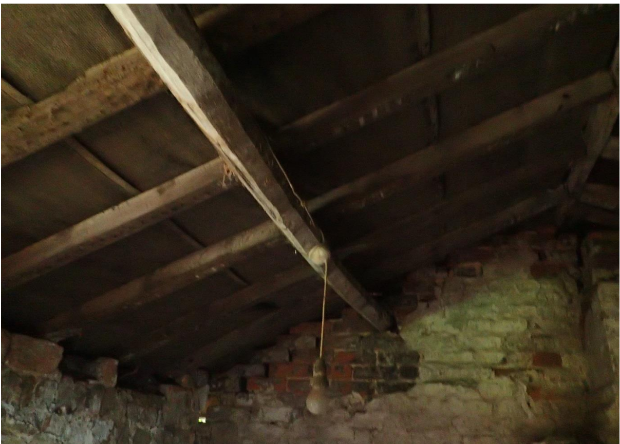
Photograph No. 10 – Detail of longitudinal distortion in purlin.
