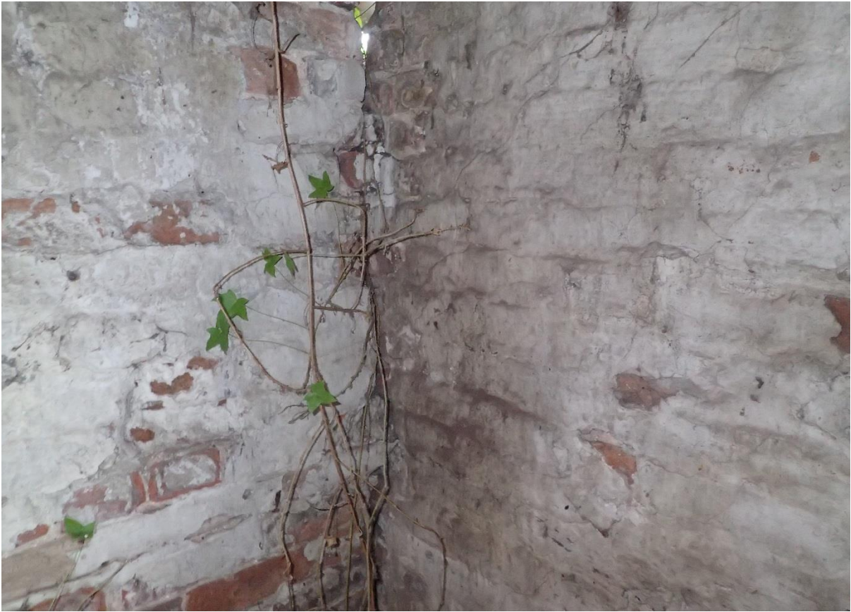
Photograph No. 1 – Detail of unbonded corner long elevation and end wall.
