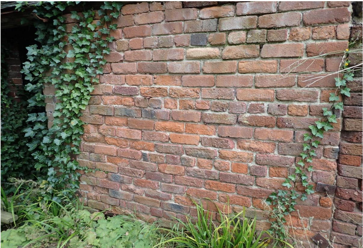
Photograph No. 8 – Typical view of external elevation show condition of brickwork and pointing.
