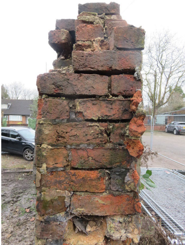
End view of the abutment of the wall where it has collapsed showing brick and a half width wall in handmade bricks.
