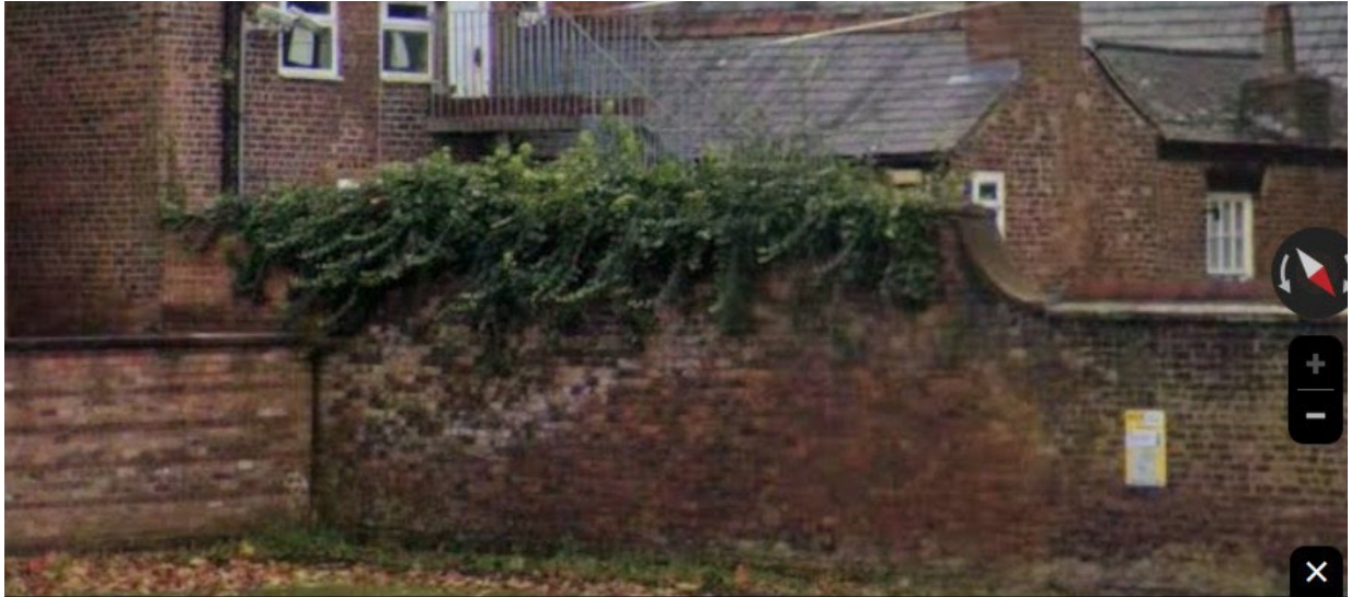
Position of wall prior to collapse.
