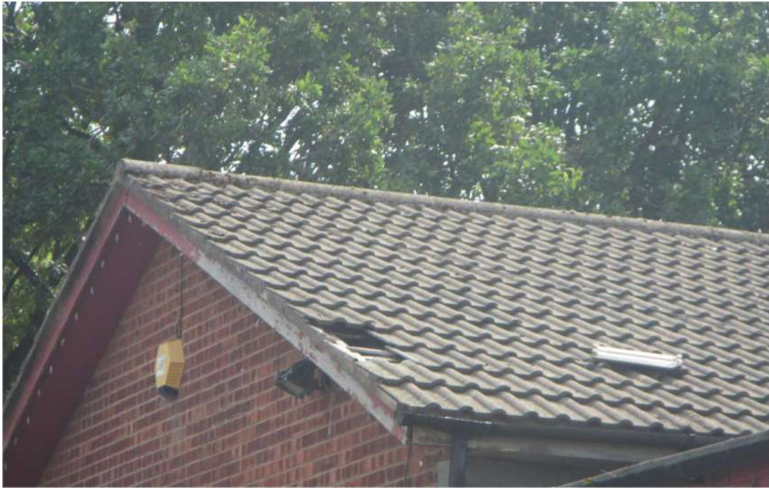
Photograph 17 – Missing tiles on the roof of Building 7.
