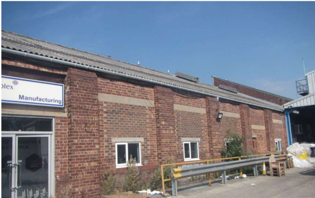
Photograph 3 – Corrugated asbestos roof on Building 1.
