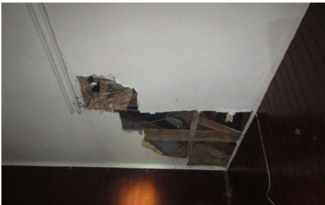
Photograph 21 – A damaged false ceiling within Building 7.
