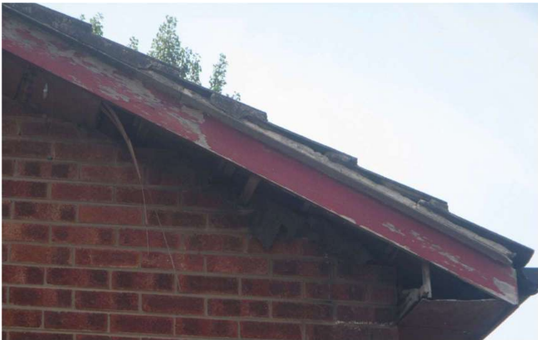
Photograph 18 – Damaged boxed soffits along the eaves of Building 7.
