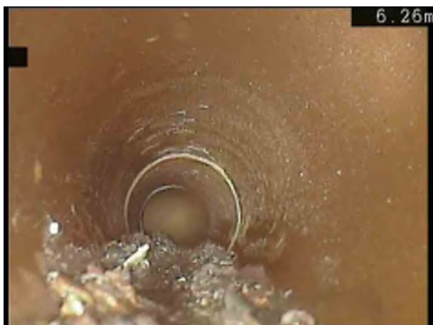
RestbendX_e1ae03dc-fa62-48d0-9cdb-468770a53eb2_20210616_144414_588.jpg, 00:00:53, 6.04 m Settled deposits, coarse, 10% cross-sectional area loss
