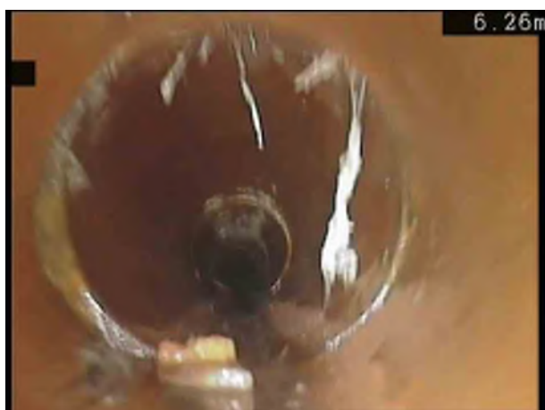
FW MH 2X_05b45c54-ffbf-4ed0-804f-946edd881bd0_20210616_145501_401.jpg, 00:00:31, 6.26 m Roots, fine at joint
