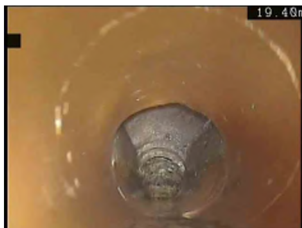
FW MH 2X_dcd94b59-a7b6-49b7-a00d-1049417c1517_20210616_145901_468.jpg, 00:01:15, 19.40 m Crack, circumferential from 9 o'clock to 5 o'clock
