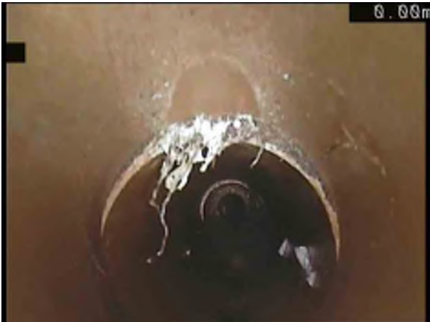
RestbendX_067135e8-2877-4bd1-905c-283d61ee4e34_2021 0616_145103_454.jpg, 00:00:20, 0.01 m Crack, circumferential at joint from 9 o'clock to 4 o'clock
