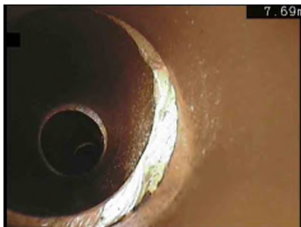
RestbendX_551fc0bd-cb36-4e11-816e-89f571abec55_20210616_144448_579.jpg, 00:01:01, 7.70 m Joint displaced, large
