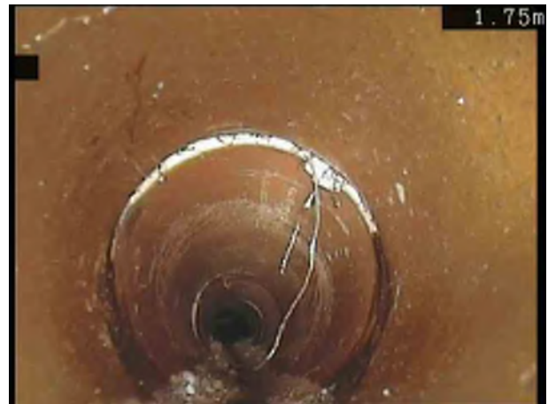
RestbendX_670773db-ba24-4e70-a202-ff0ea71a3075_20210616_144039_985.jpg, 00:00:25, 1.75 m Roots, fine at joint
