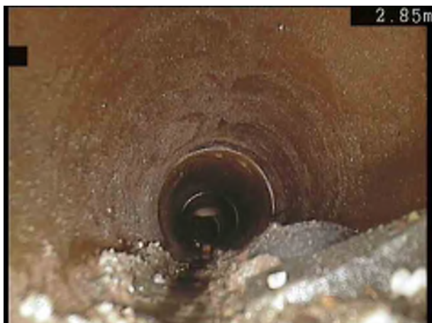
RestbendX_a1255de8-41b1-417e-bfa2-59b1900ebc1c_20210616_144324_703.jpg, 00:00:38, 2.85 m Settled deposits, coarse, 15% cross-sectional area loss
