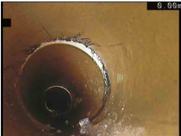
RestbendX_27f34987-24cf-470e-85e7-e43a7974c5d0_20210616_144016_834.jpg, 00:00:12, 0.01 m Roots, fine at joint
