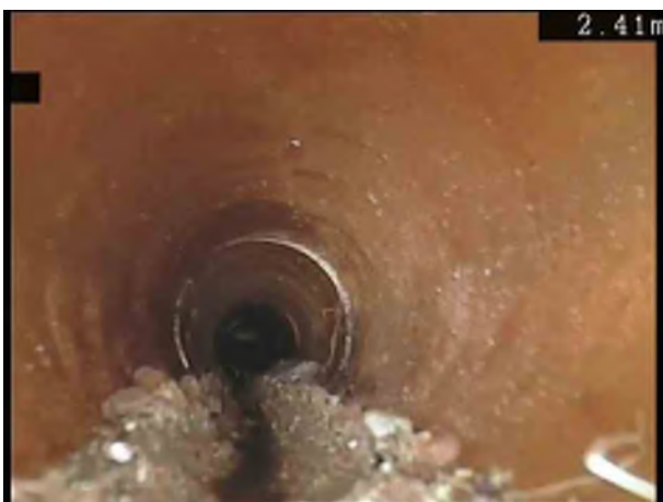
RestbendX_0f3820d8-099e-425e-9139-fdf29d5a9806_20210616_144256_545.jpg, 00:00:32, 2.41 m Settled deposits, fine, 15% cross-sectional area loss
