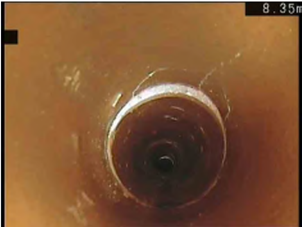
RestbendX_9fea196c-3957-46a2-a91d-e2bb84135b2c_20210616_144522_065.jpg, 00:01:13, 8.35 m Crack, circumferential from 11 o'clock to 2 o'clock
