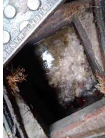
FW MH1 blocked
