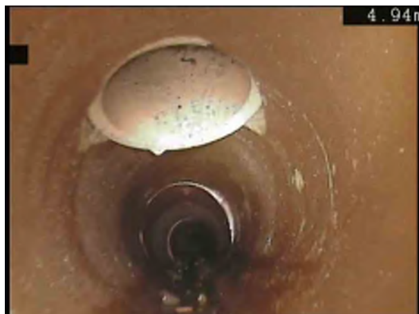
RestbendX_4feb9845-e82f-488f-ba6b-d6561b4100a5_20210616_144353_230.jpg, 00:00:48, 4.94 m Connection defective, position incorrect at 12 o'clock, diameter: 100mm
