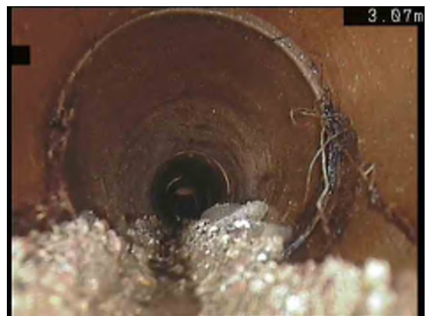
RestbendX_e97dd8f5-d18d-47f9-9da7-c47fa0386f7b_20210616_144309_657.jpg, 00:00:34, 2.85 m Roots, fine at joint
