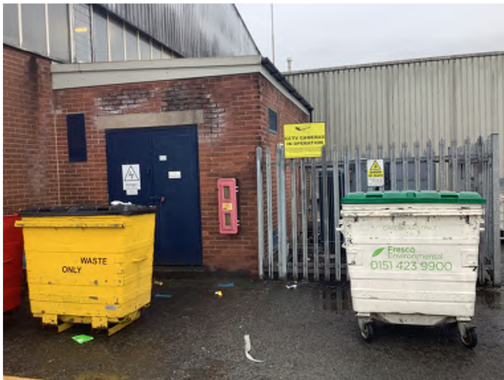
Photo Plate No. 21: Electrical Sub station
