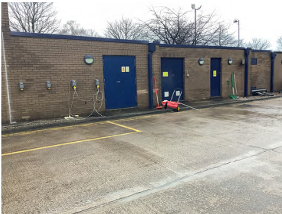
Photo Plate No. 01: Electrical Substation and Gas Plant (Feature 1)
