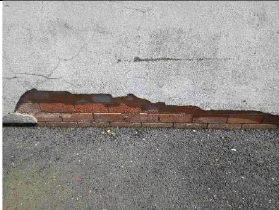
Photograph 11: Cracked and missing rendering on south-western elevation of B1
