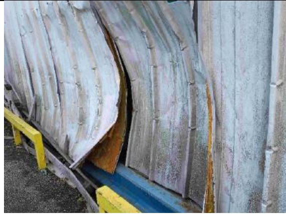
Photograph 12: Misshapen cladding of north-western elevation of B1
