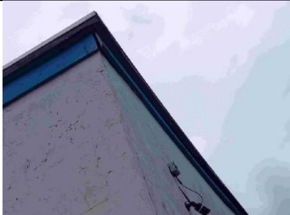
Photograph 17: Gaps between facias and walls on B2
