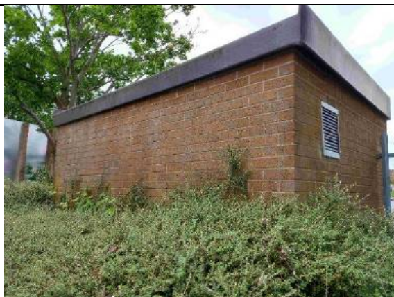
Photograph 20: Gas governor station (TN3)
