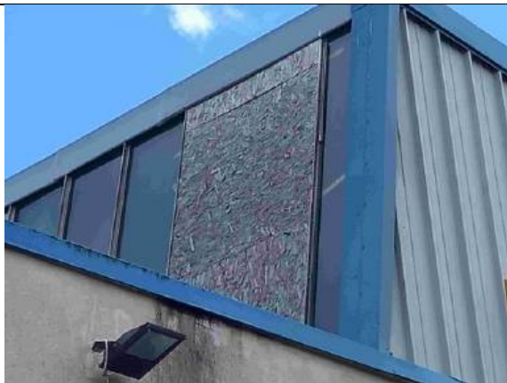
Photograph 13: Boarded window on north-western elevation of B1
