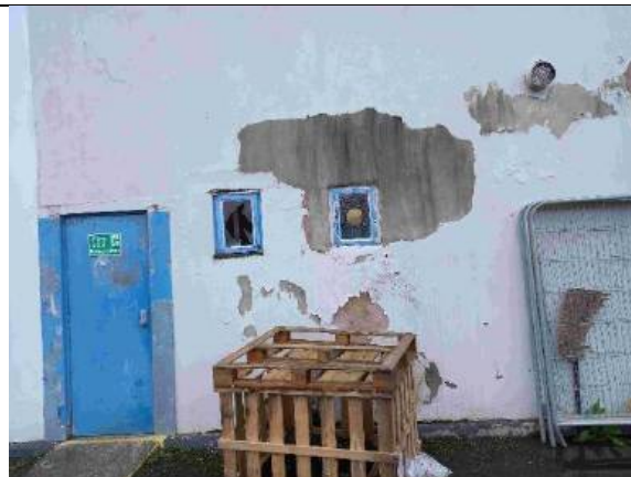
Photograph 16: Crack and missing rendering and broken windows on south-eastern elevation of B2
