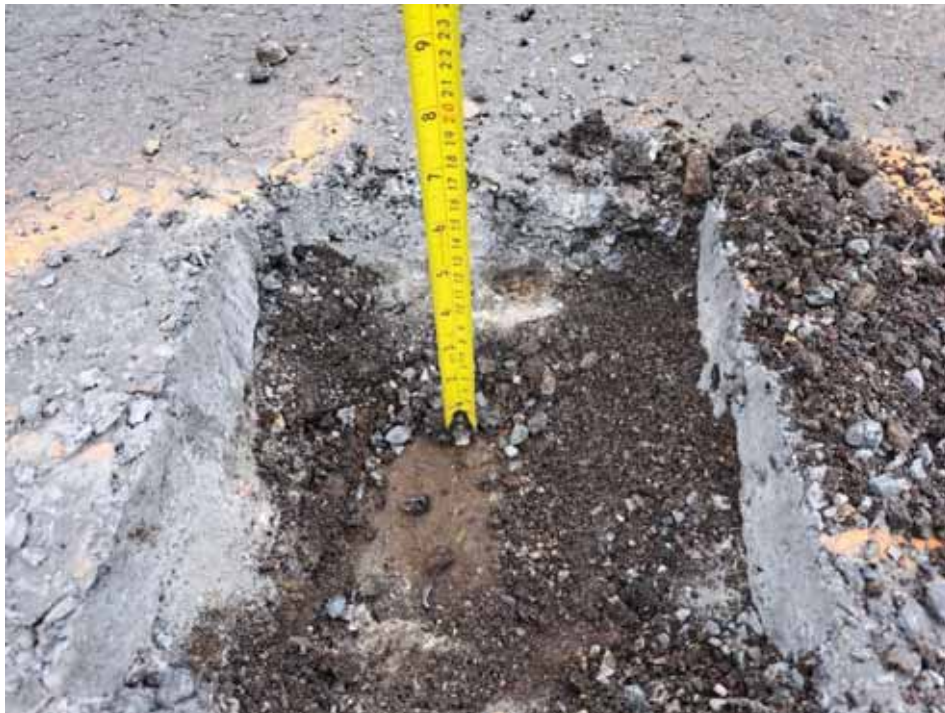
Photograph 23 WS111 obstruction beneath tarmacadam hardstanding
