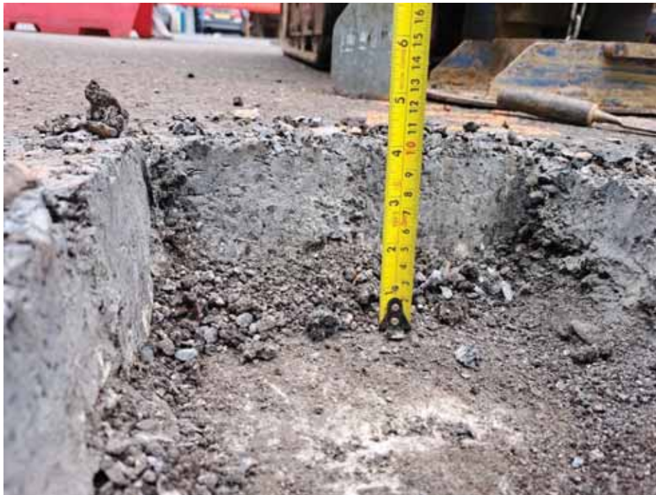
Photograph 25 WS112 obstruction beneath tarmacadam hardstanding
