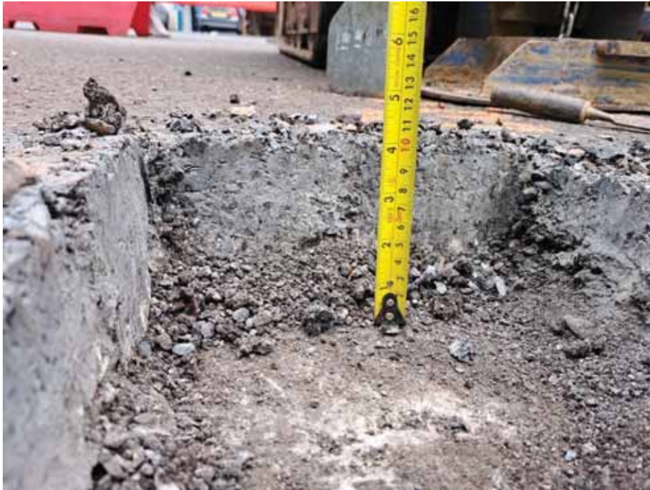
Photograph 25 WS112 obstruction beneath tarmacadam hardstanding
