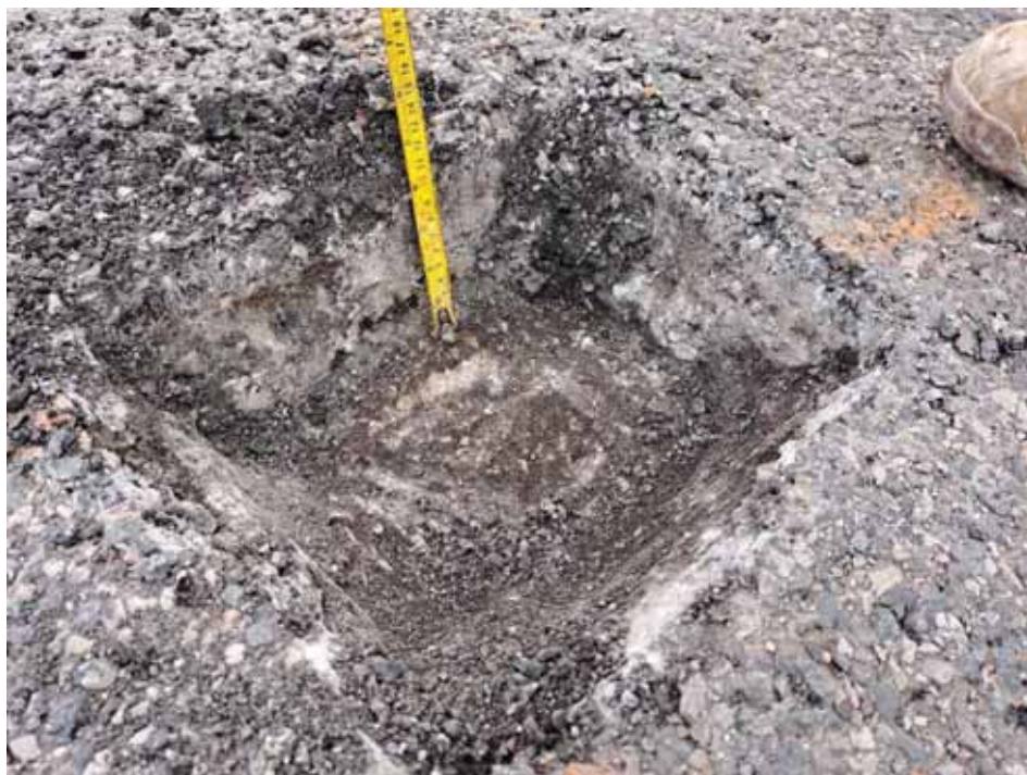
Photograph 14 WS107 obstruction below tarmacadam hardstanding
