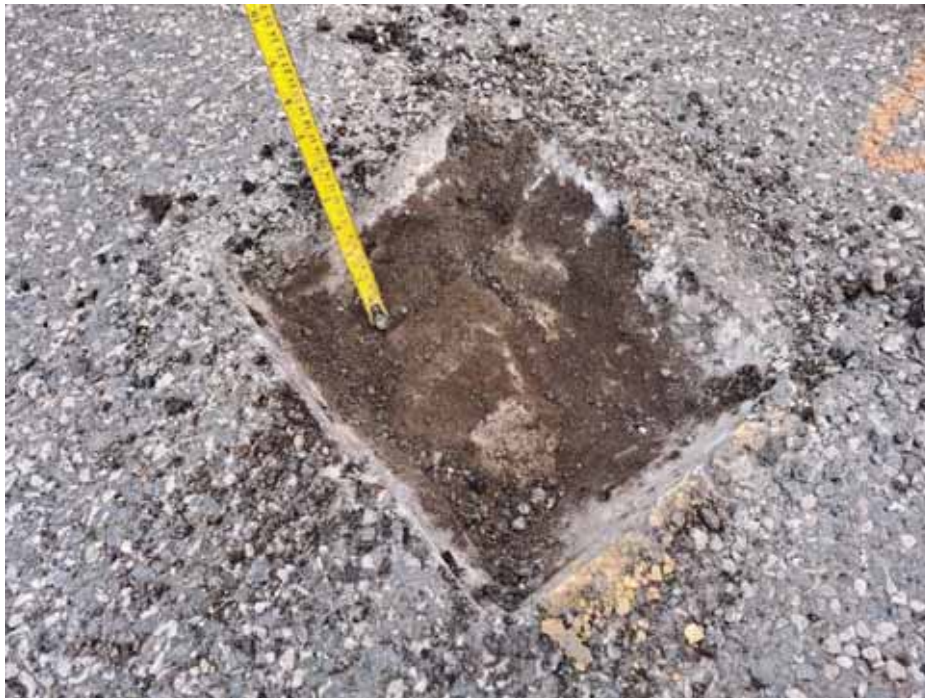
Photograph 17 WS109 showing obstruction below tarmacadam hardstanding
