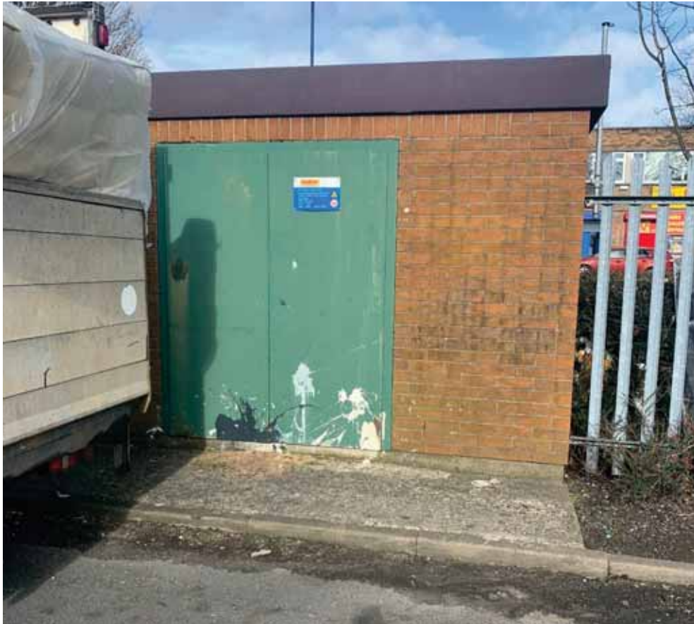
Photograph 11 Gas governor adjacent to the electricity sub-station.
