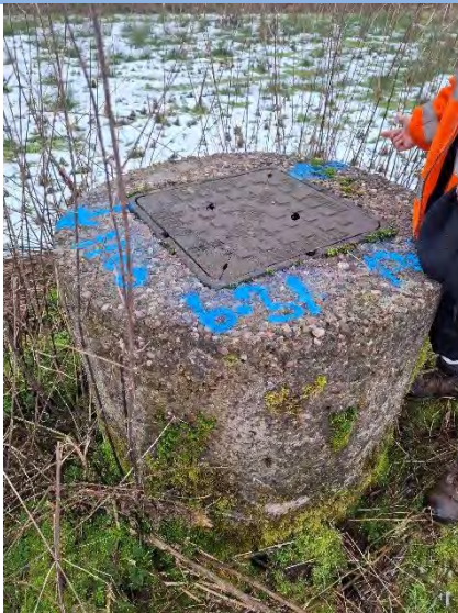
Photograph 3: Above ground manhole
