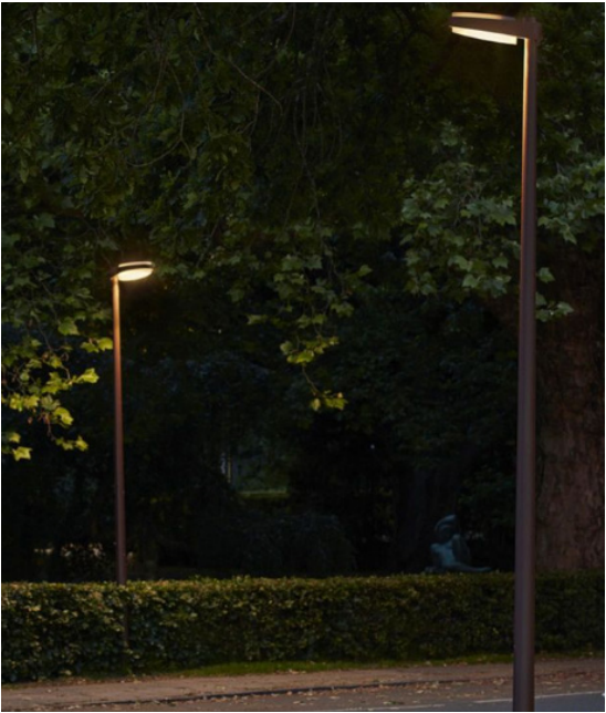
Car park lighting architectural lighting columns
