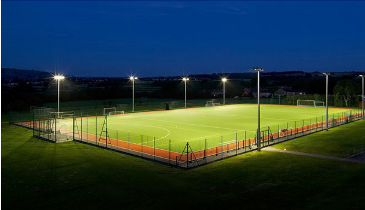
Column mounted floodlights
