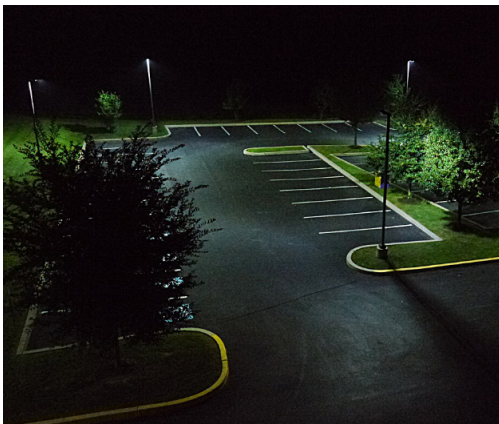
Column lighting for carpark
