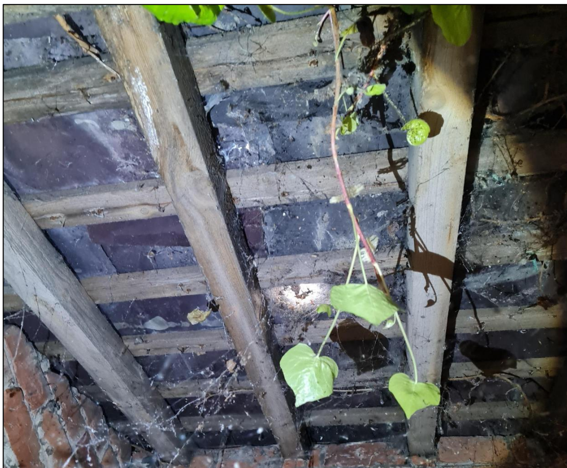
Plate 6 – Slipped slates evident on roof of outbuilding
