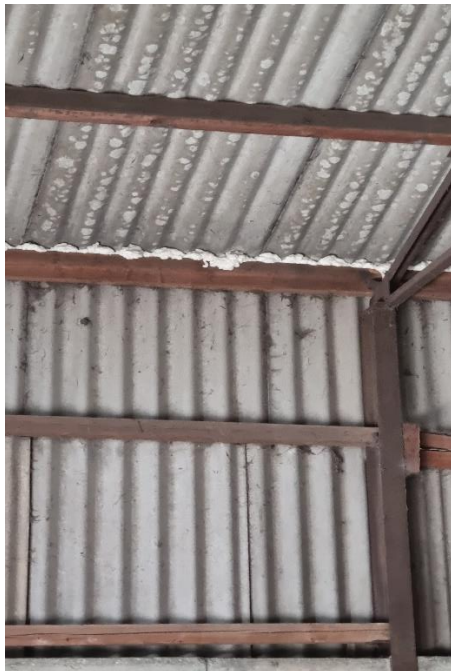
(Foam filler – gaps at the Eaves)
