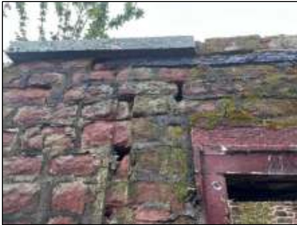
Figure 25: Voids in the walls of the building.
