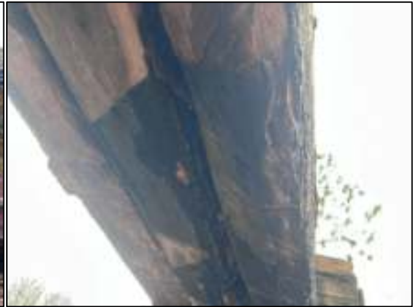
Figure 26: Gaps between lintels.
