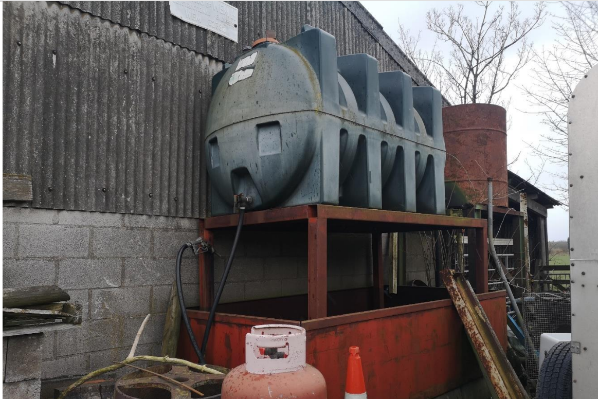
PLATE 3 ABOVE GROUND SOTRAGE TANK ADJACENT TO FARM BUILDING
