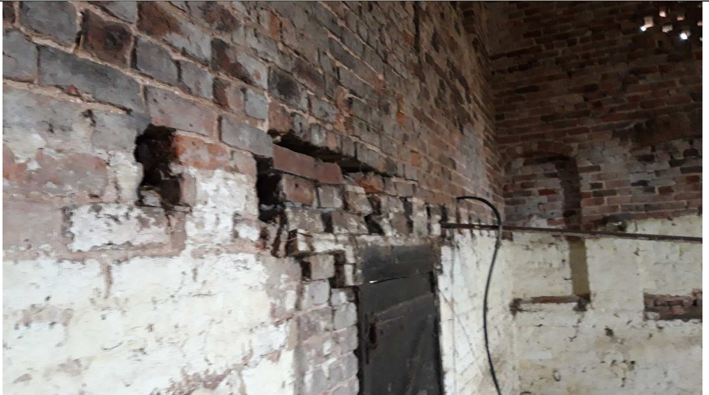
Building F8 –Masonry Damage Above Lintel to South Wall in Western Room
