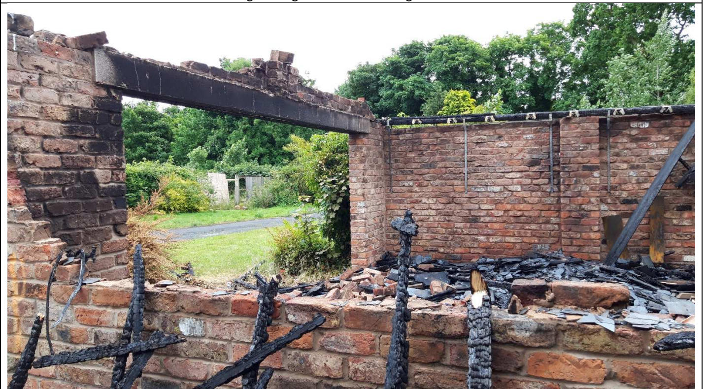
Building F9 – Severe Fire Damage to Garage
