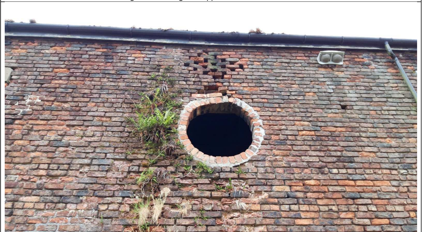
Building F8 – Damage to External Masonry at Eastern End of North Elevation
