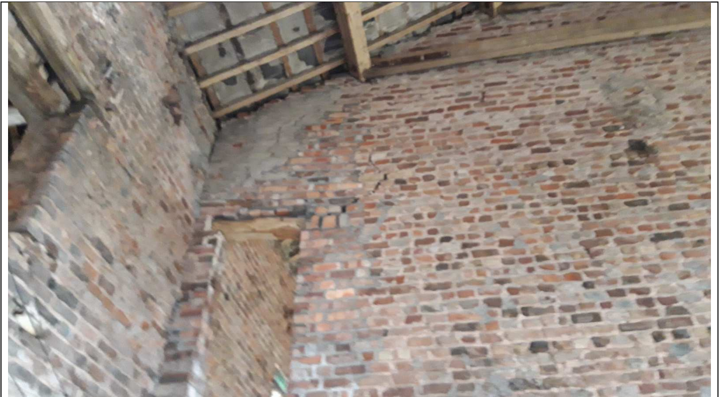
Building F8 – Cracking to Propped Partition Wall at East End
