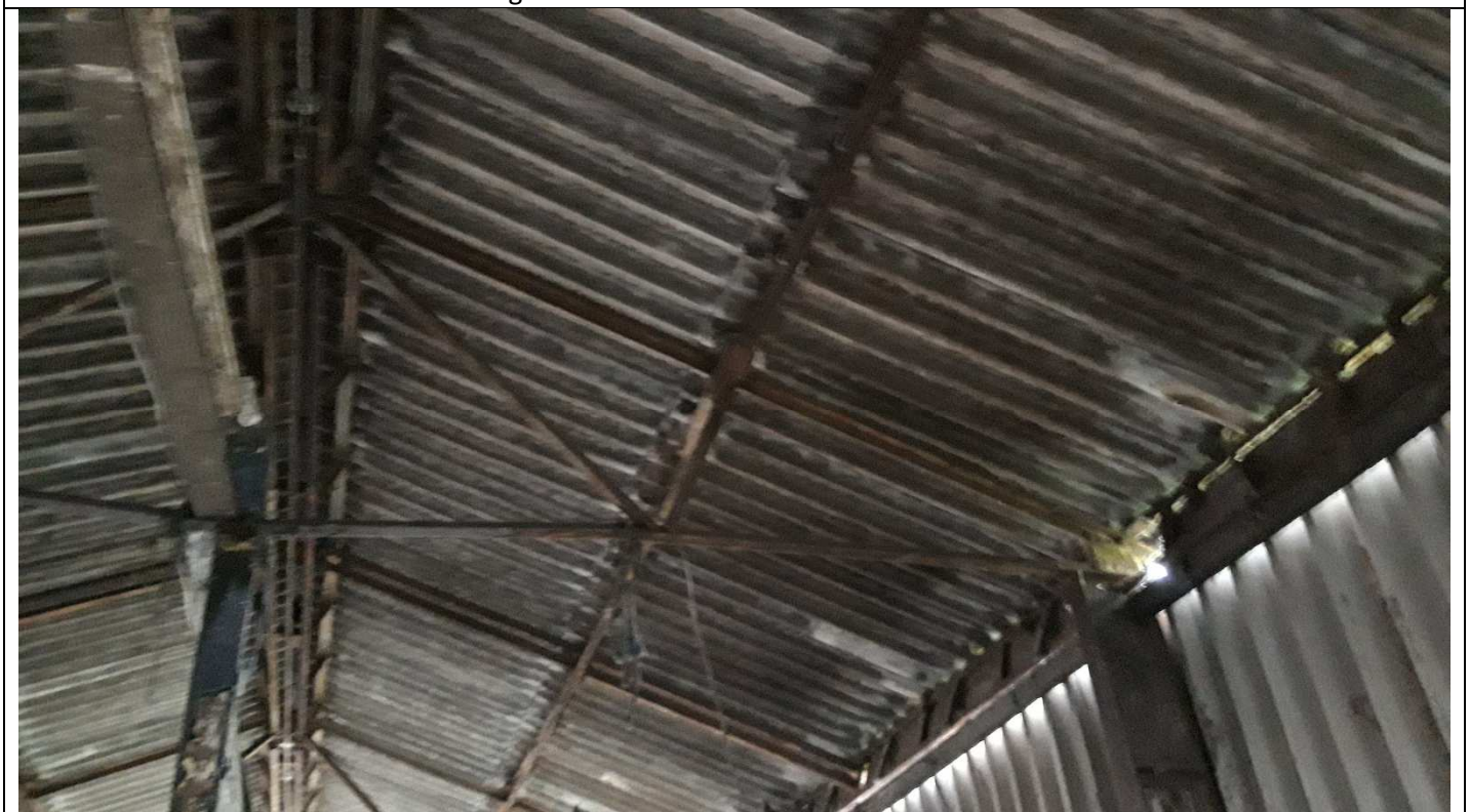
Building F5 – Detail of Framework to South (dilapidated) Storage Shed
