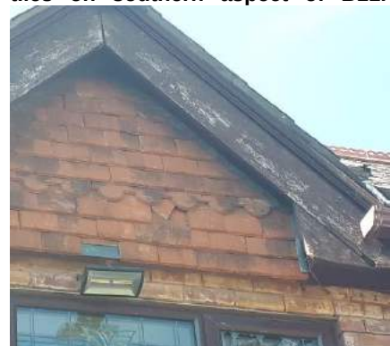
Photograph 31: Gap in clay hanging tiles on southern aspect of B11.
