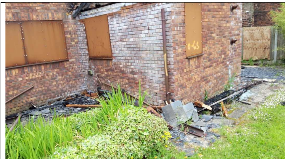
Photo 04: Fire debris to rear of House
