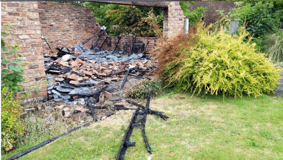
Photo 03: Fire damage to garage
