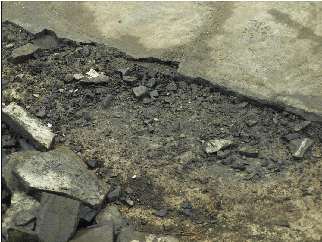
Plate 37: Bitumen covered floor
