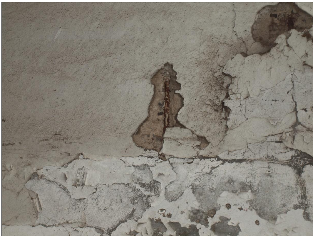
Plate 19: Detail of rebar visible within concrete
