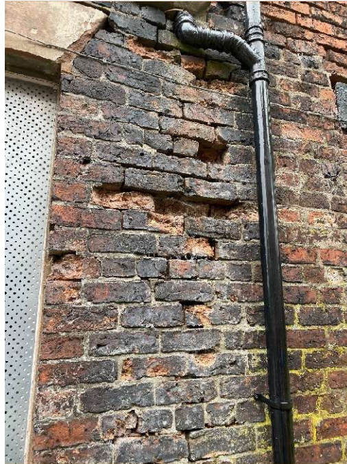
Plate 3 – Spalled brickwork and open joints to south elevation. Deterioration is aligned where end cap is missing from the guttering.
