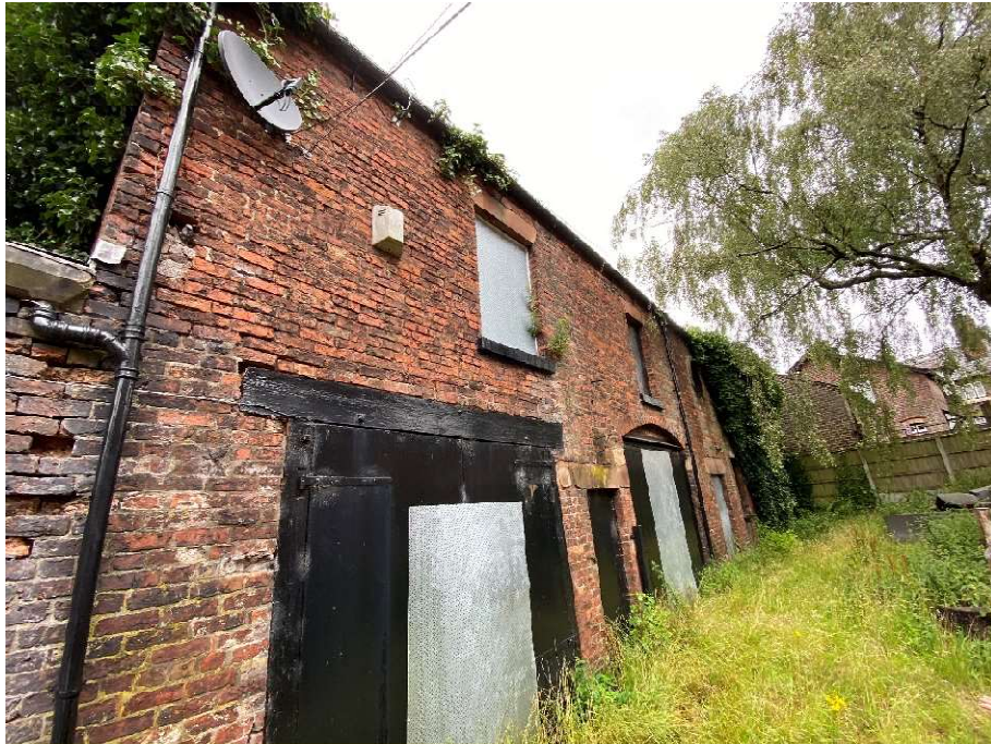
Plate 1 – south elevation of the stable block with satellite dish to left and vegetation growth to the right (east) end.
