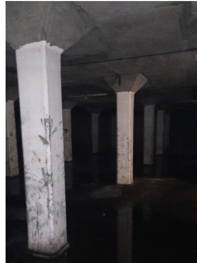
Flooded Interior and Columns
