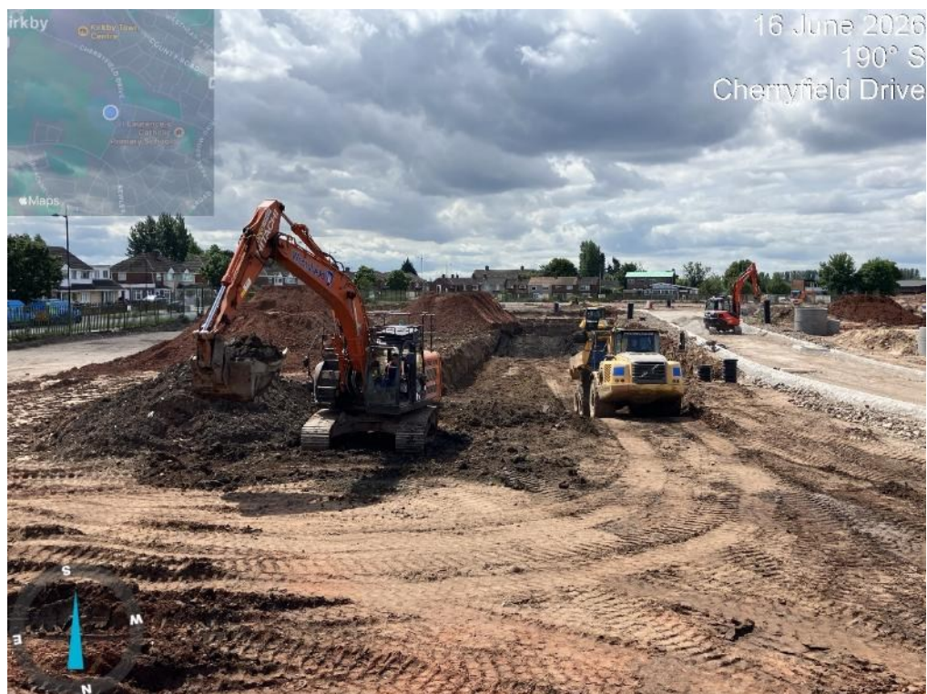
Plate 4 Risk to Infrastructure
