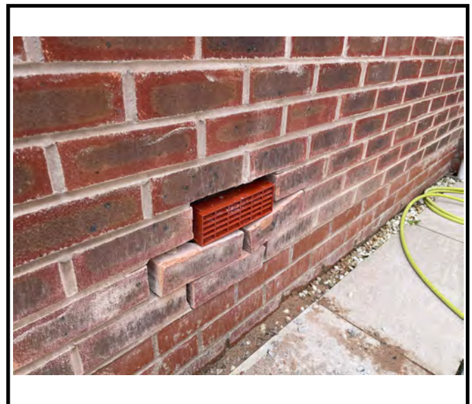
An air brick installed around the external perimeter of the Conservatory.
