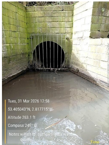
Photo 11: Outflow, poor water quality (SJ 45734 90114)
