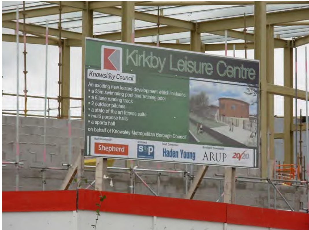
Photo 21: Close up of sign shown in Photo 20
