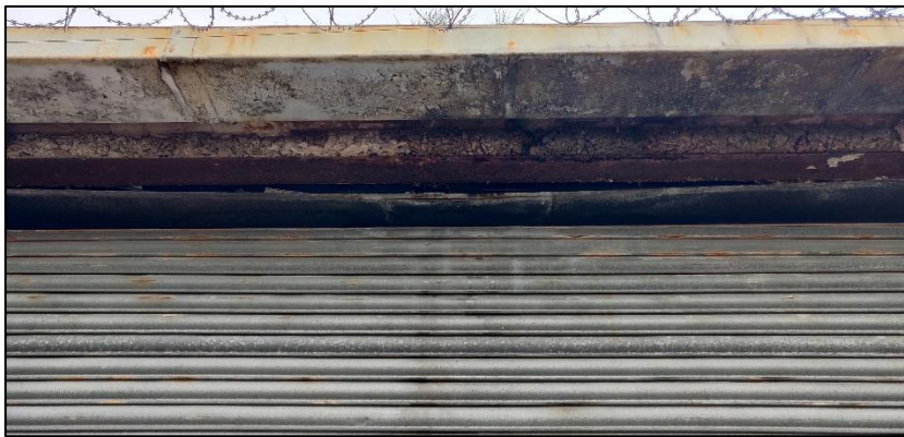
Photograph 23 showing a gap above one of the metal shutters
