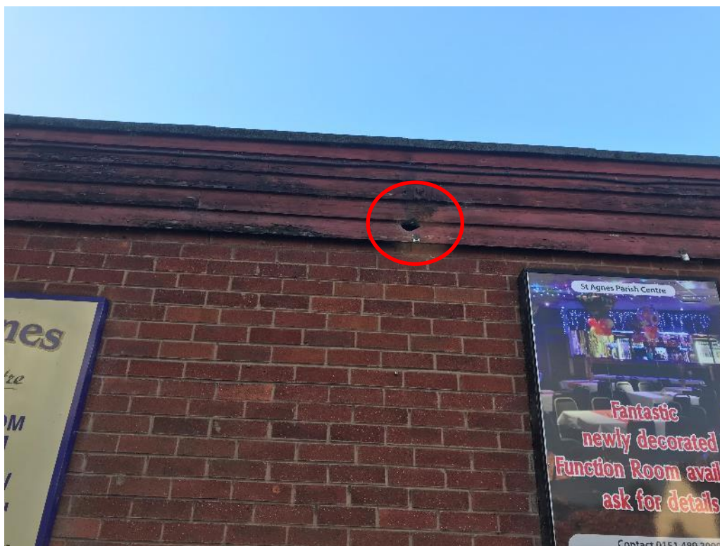
Plate 5 – Typical gap in the cladding on the northern elevation
