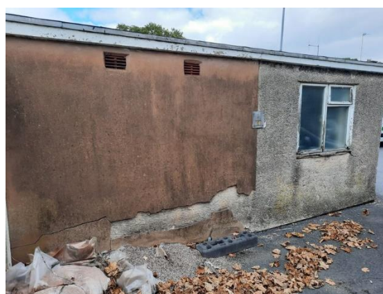
Plate 4.9: Peeling Render and Rotten Window Frame to South-east of Building B2.
