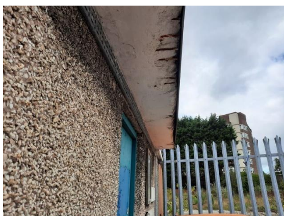
Plate 4.8: Degraded Concrete and Gap Around Fascia to North-west of Building B2.
