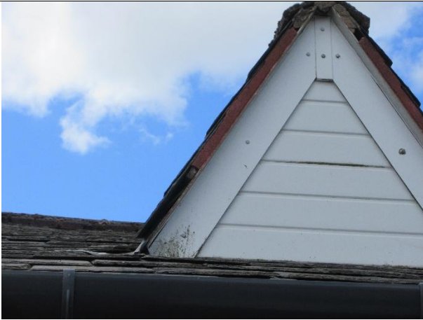
Photo 25: Missing mortar at roof verge on dormer at garage
