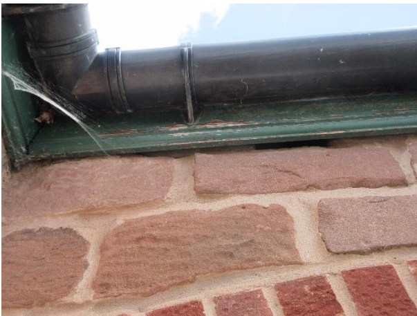
Photo 9: Gaps at timber fascia at cottage
