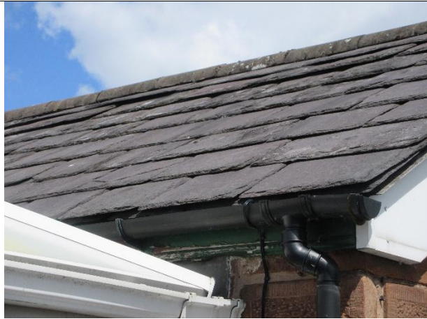
Photo 8: Roof of cottage showing gaps / potential roost feature at lifted slates
