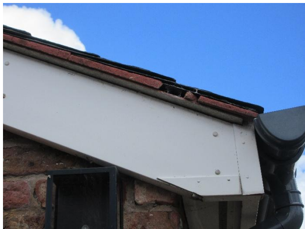
Photo 24: Missing mortar at south-facing gable end of the garage
