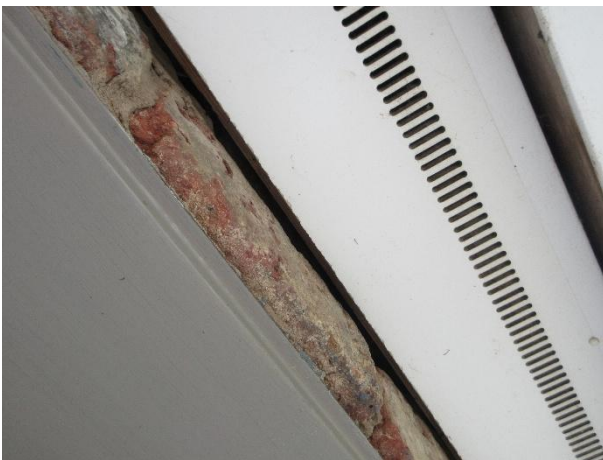
Photo 23: Gap above garage door
