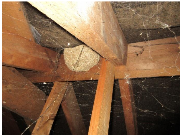
Photo 12: Roof void at cottage showing wasp nest
