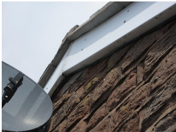
Photo 10: Gaps at PVC fascia at cottage
