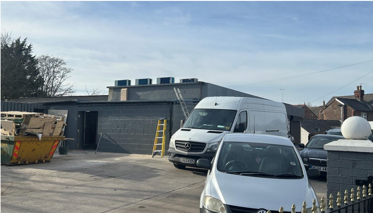
Figure 2: Photograph showing installed units
