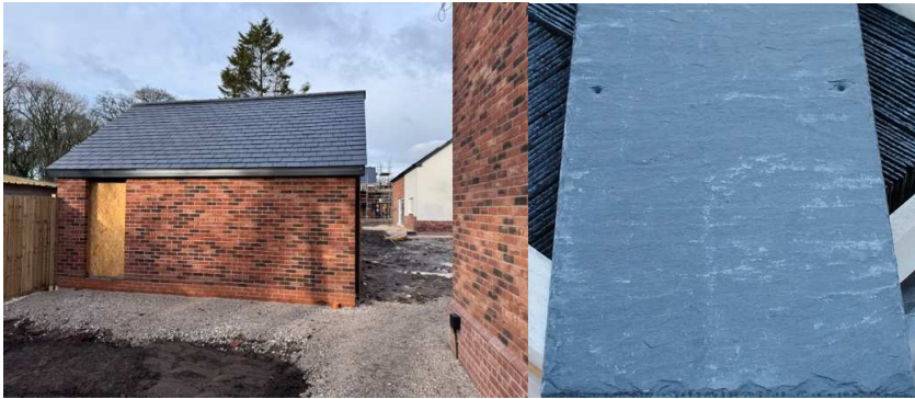
Windows – White UPVC with Georgian bar (Efficiency Rating – A)
